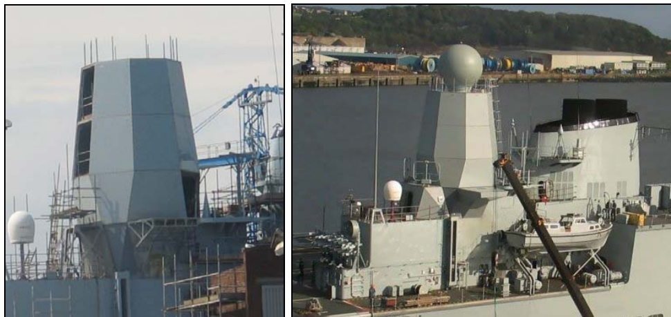
Figure 7: (a) Initial mast mounting on HMS Ark Royal (b) Mast with panels in-situ
