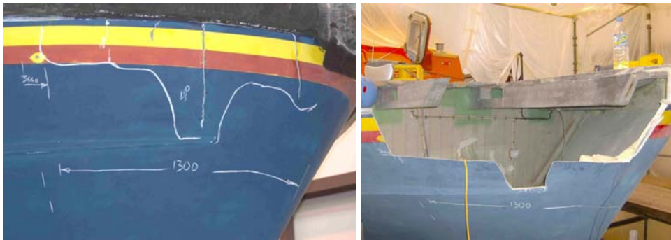
Figure 3 – Damage marked up after inspection and with damaged material removed
